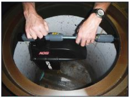
ECHO with installation bar mounted on manhole frame
