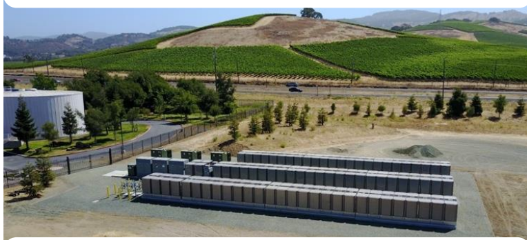
Healthcare Data Center 4.75 MW Installation
