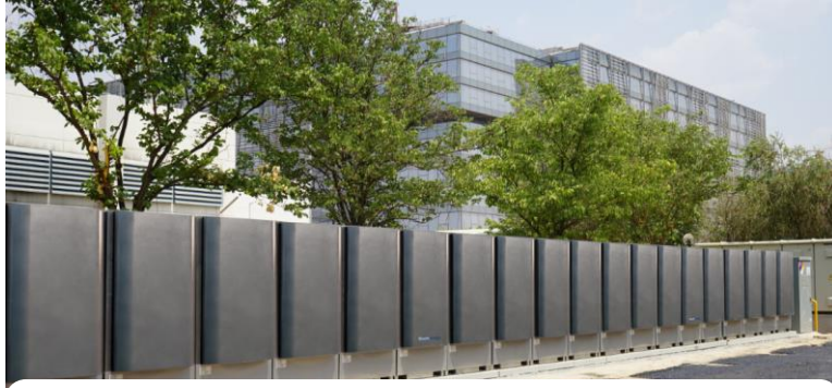
Semiconductor Microgrid 2.5 MW Installation
